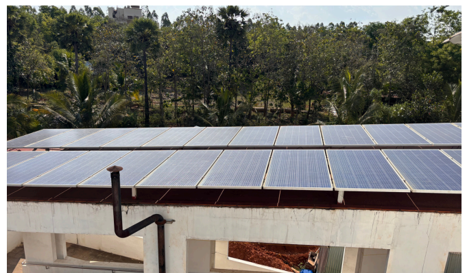
Image 4: Rooftop solar installation
